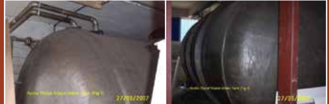
Acidic Glycol Waste Water Tank in Singapore
